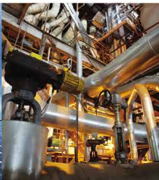
Oil & Gas Plant
