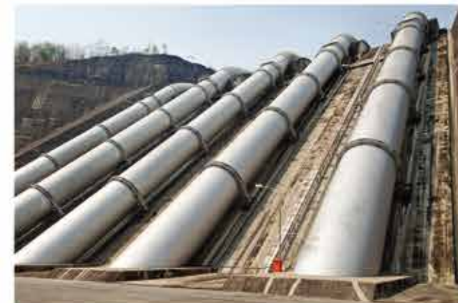
Water pipeline to Hydro-Electric power station
