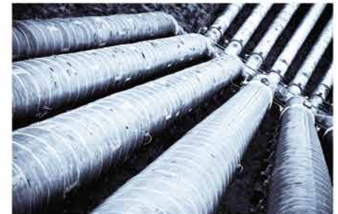
Water pipeline to Hydro-Electric power station
