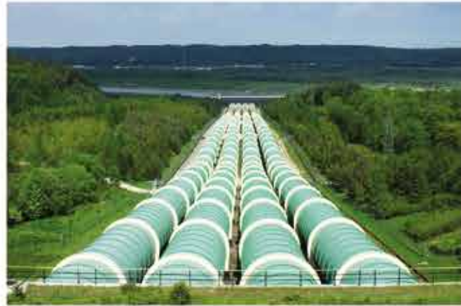
Gigantic water pipes of a power plant
